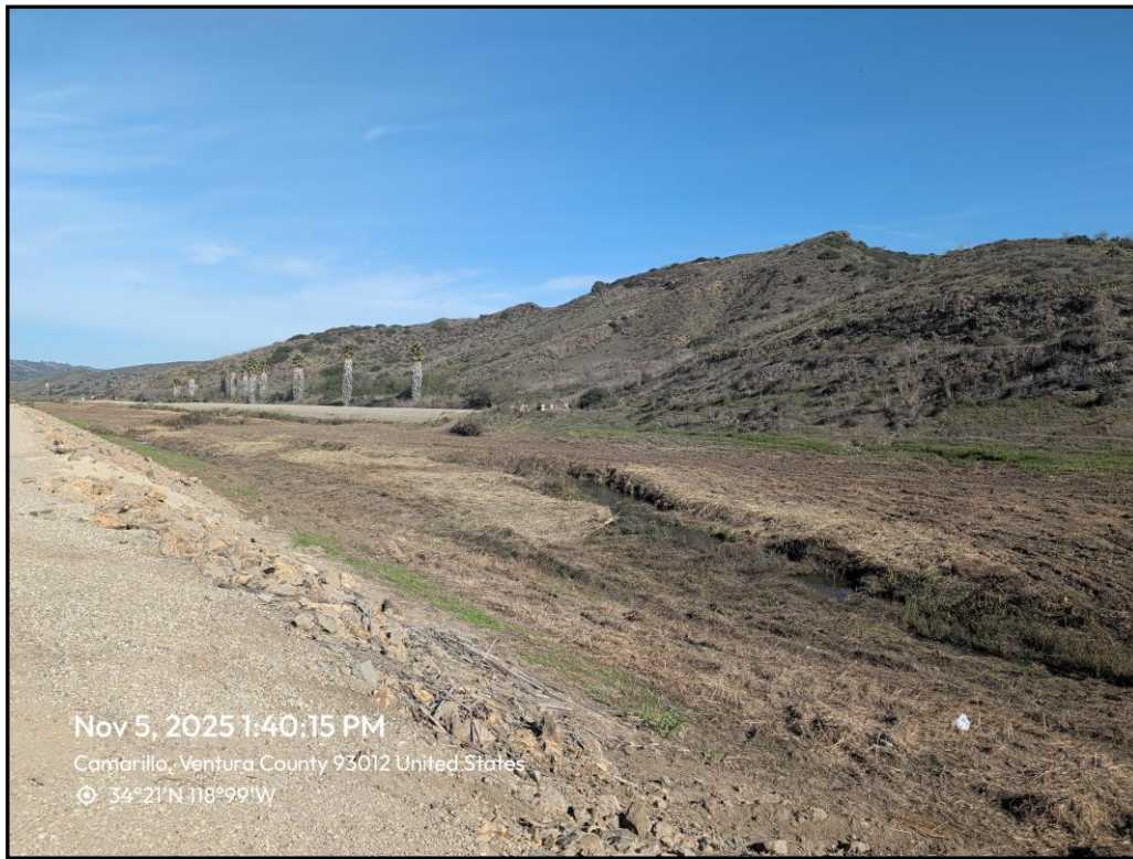
Photo 2. Looking upstream (northeast) from the west levee access road near Highway 101 following project activities, November 5, 2025.
