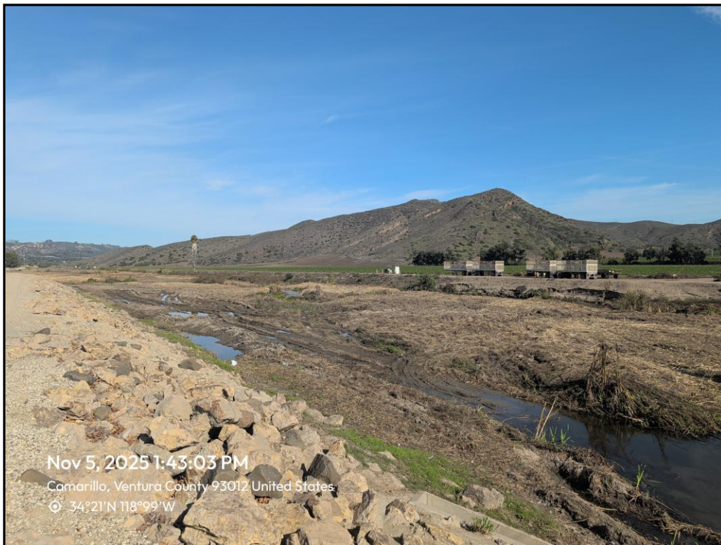
Photo 6. Looking upstream (northeast) from the west levee access road following project activities, November 5, 2025.
