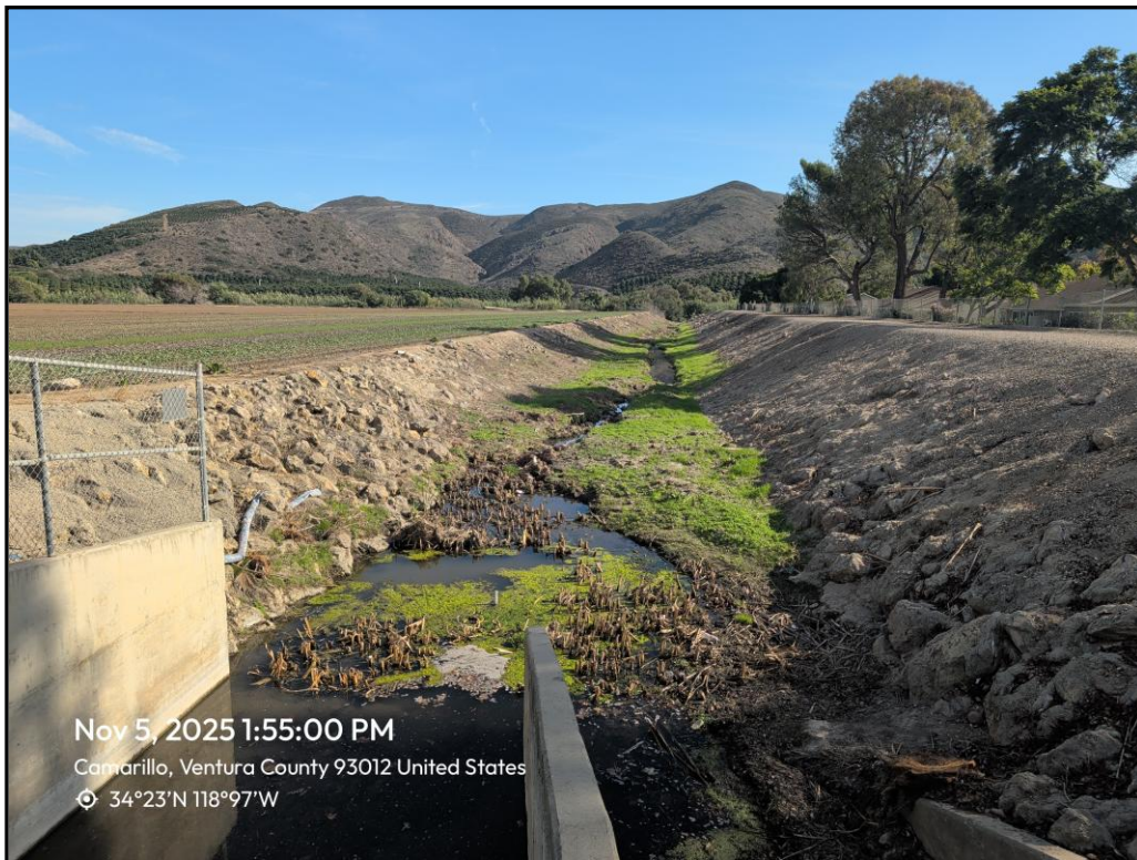
Photo 17. Looking downstream (southeast) from outlet of Upland Road Drain, near Santa Rosa Rd. following the completion of project activities, November 5, 2025.
