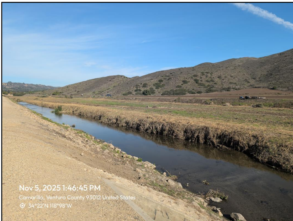
Photo 10. Looking upstream (northeast) from the west levee access road near Mission Oaks Drain following project activities, November 5, 2025.
