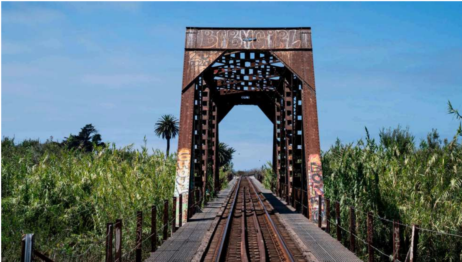
A railroad trestle runs over the Ventura River estuary, with stands of Arundo along the banks. Kitra Cahana/Undark
